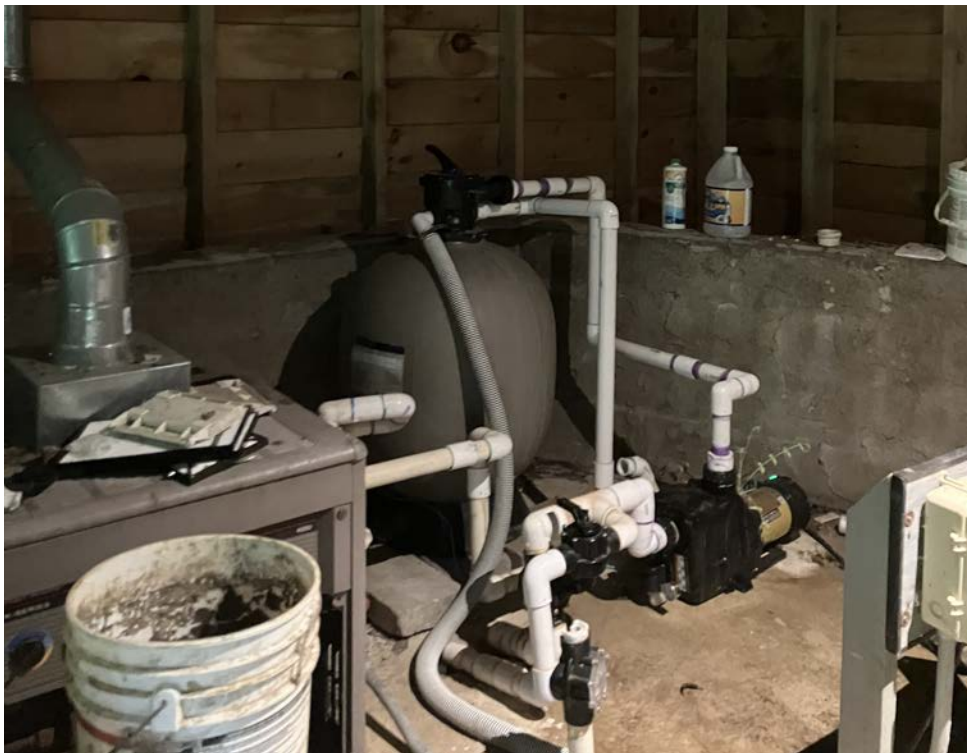
Accessory Structure View of Interior Pool Equipment
