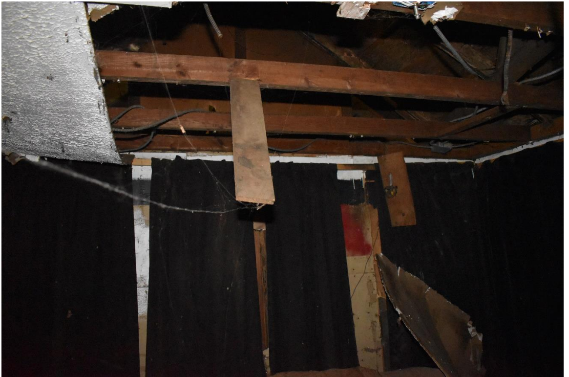
9. View to the north of the northern addition. Lumber indicates a mid-late 20 th century construction date.
