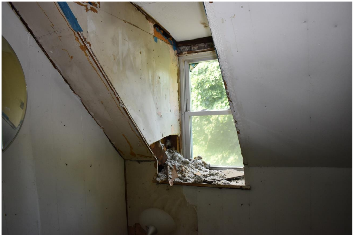
16. View to the southwest of the southern dormer. Note the significant water damage.
