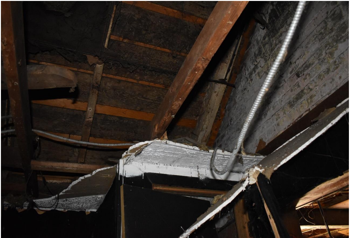
10. The interior of the northern addition has completely deteriorated. View to the southeast.
