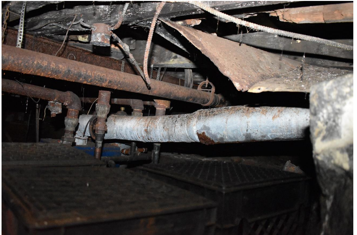
20. Pipes and mechanicals are located in the basement of the structure.
