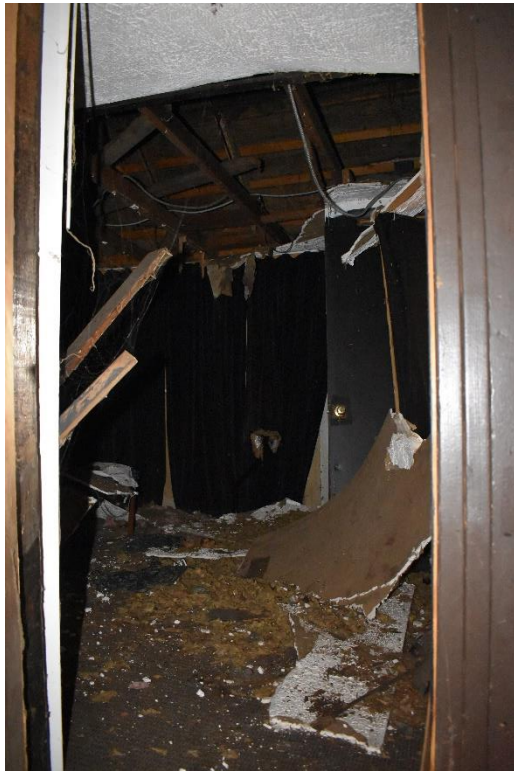
5. View to the northeast of the northern addition. The interior of this space is deteriorating.
