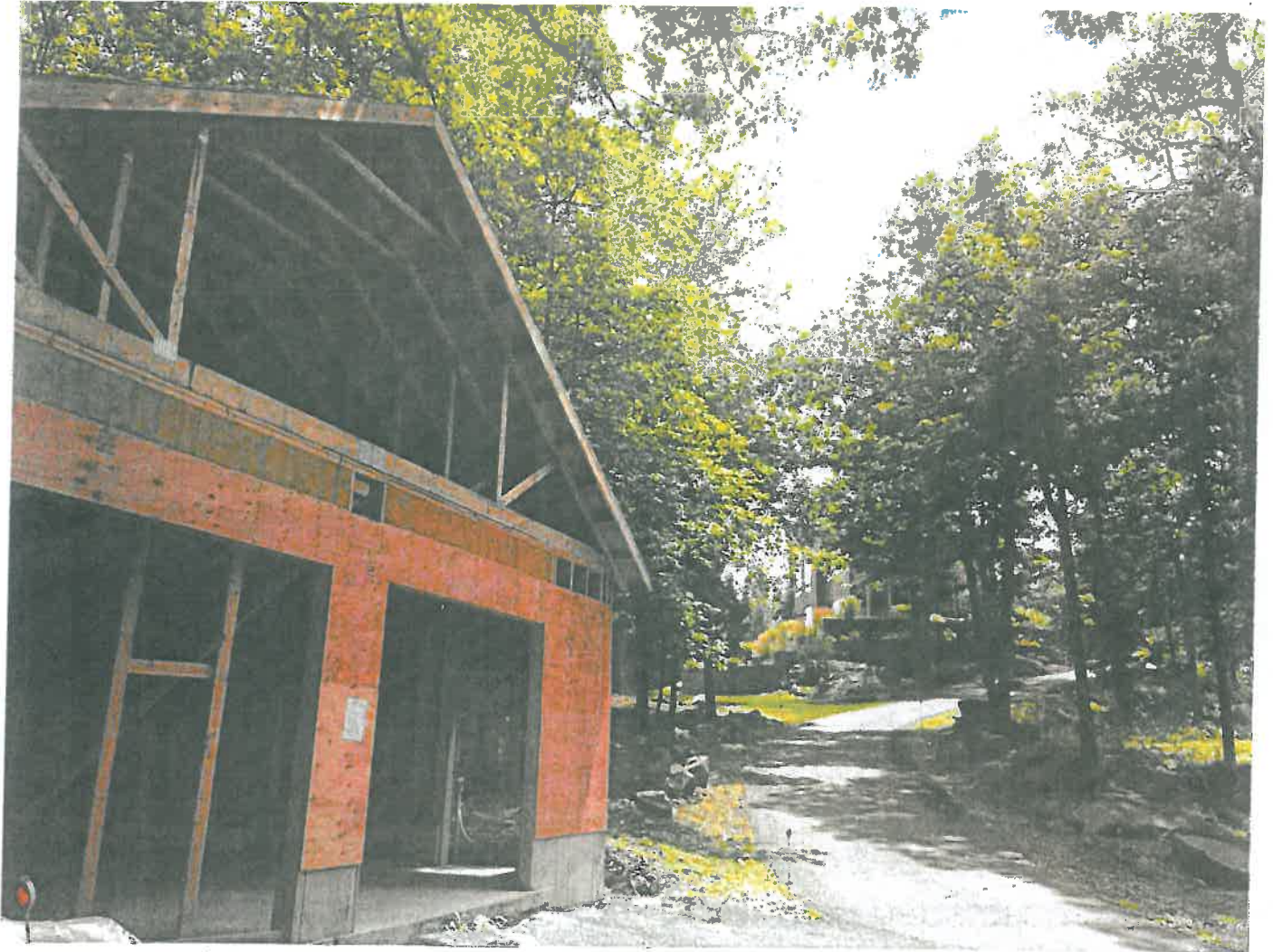
Partially constructed barn with house in upper background, note large trees surrounding the area.
