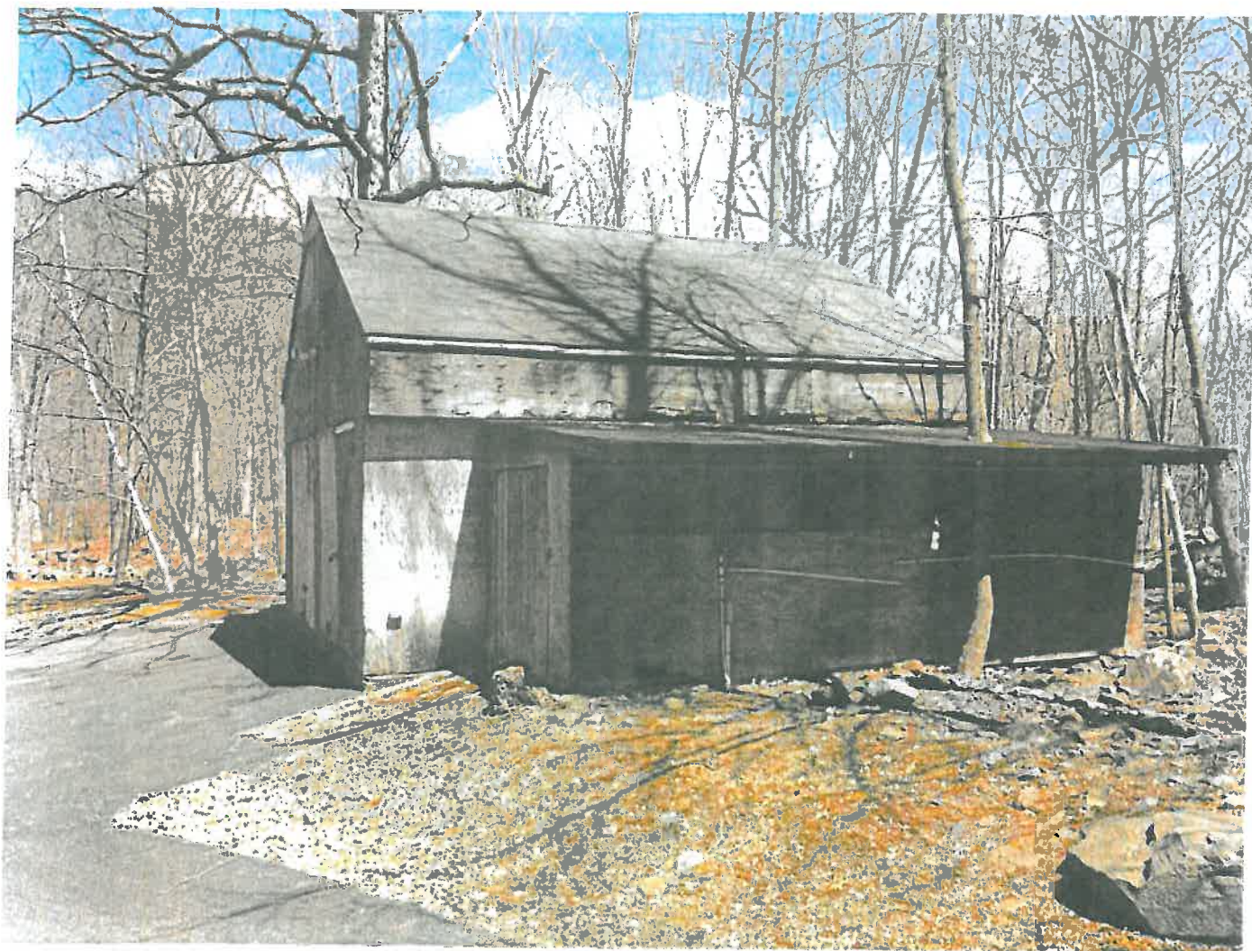
View of barn from south, extensive rot visible.
