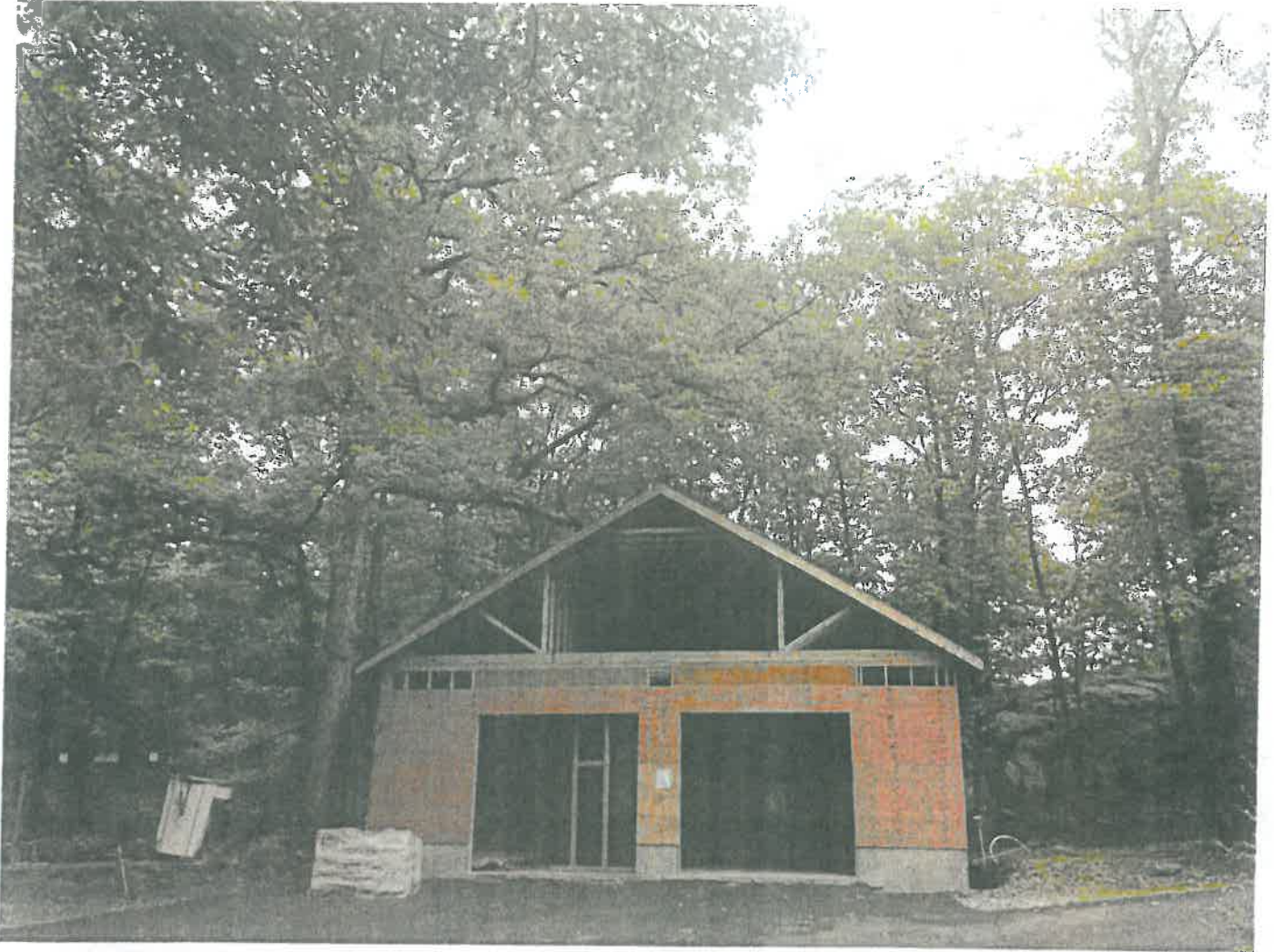
Facade of partially constructed garage (substantially similar footprint and dimensions to previously existing barn). Tall trees in surrounding area.
